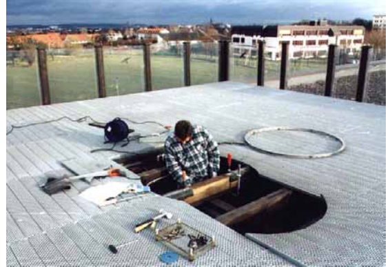
Installation of a RST 072 \varnothing 1.2 m in an OATS next to Frankfurt
